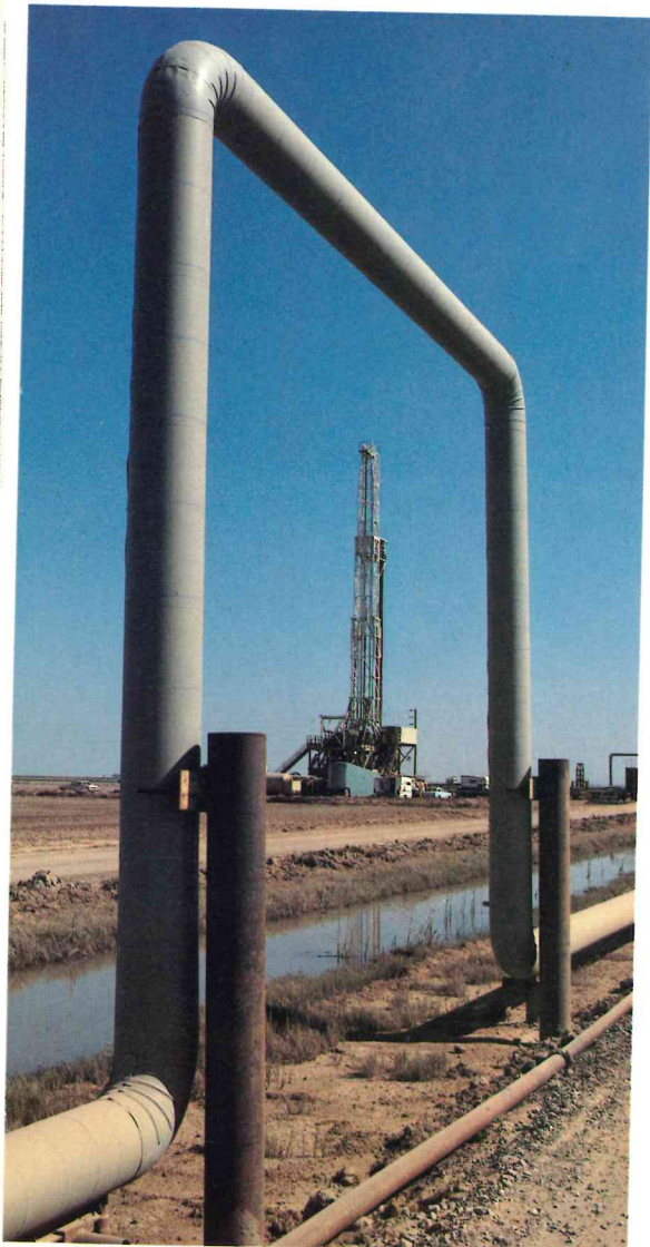
Loops in the steam pipeline from an Imperial Valley well in the Niland area are designed to accommodate expansion due to temperature changes.
