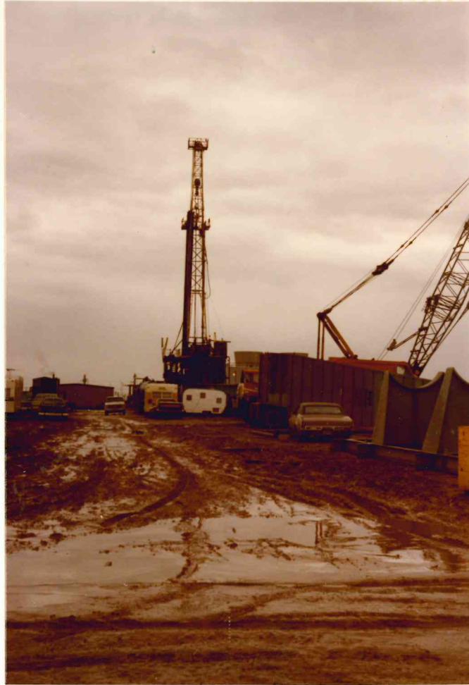
Construction of the Brawley Geothermal Power Plant Steam Gathering System began during November, 1979. Before the wells could be used for power production, they had to be worked-over. A drill rig was used to clean out the wells and check their production in sometimes awful conditions.
