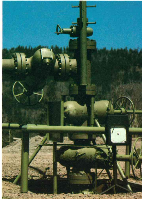
Valves control the flow of geothermal fluids which are brought to the surface through wells drilled deep into the earth. Pipeline and wellhead equipment is painted to blend with the local environment.
