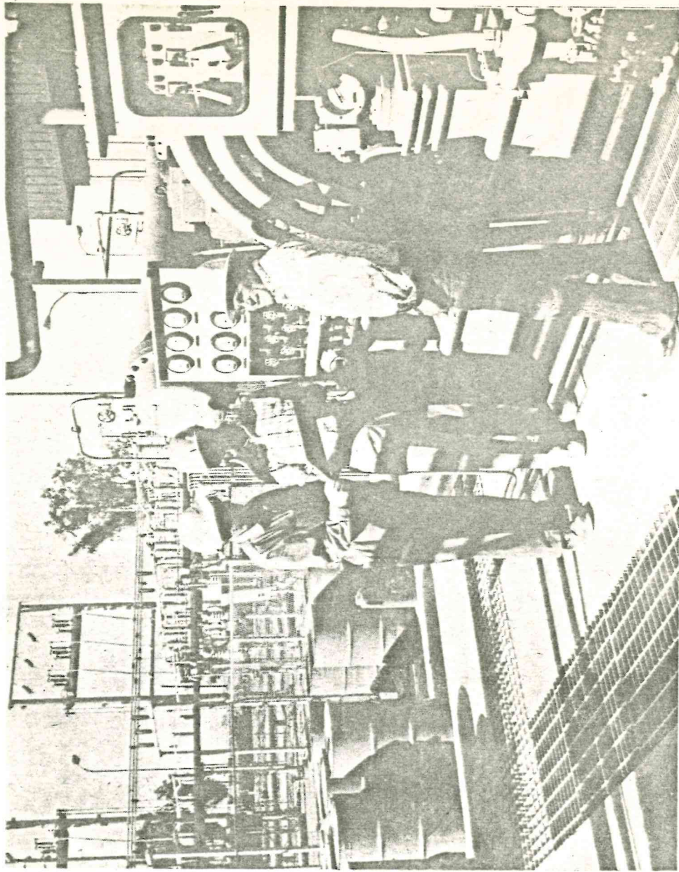
POWER TO IID — Experts at the Geothermal Test Facility north of Brawley watch and wait as the installation, the first to utilize a flash system in the U.S., feeds 1.5 megawatts of electricity into nearby
